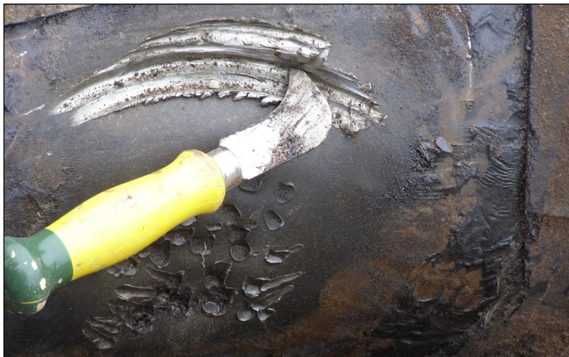
Figure 1: A knife inserted into the hole in the pipeline, created by a drill bit. The primary cause of the incident was failure to have the pipeline located by calling BC One Call prior to drilling.
